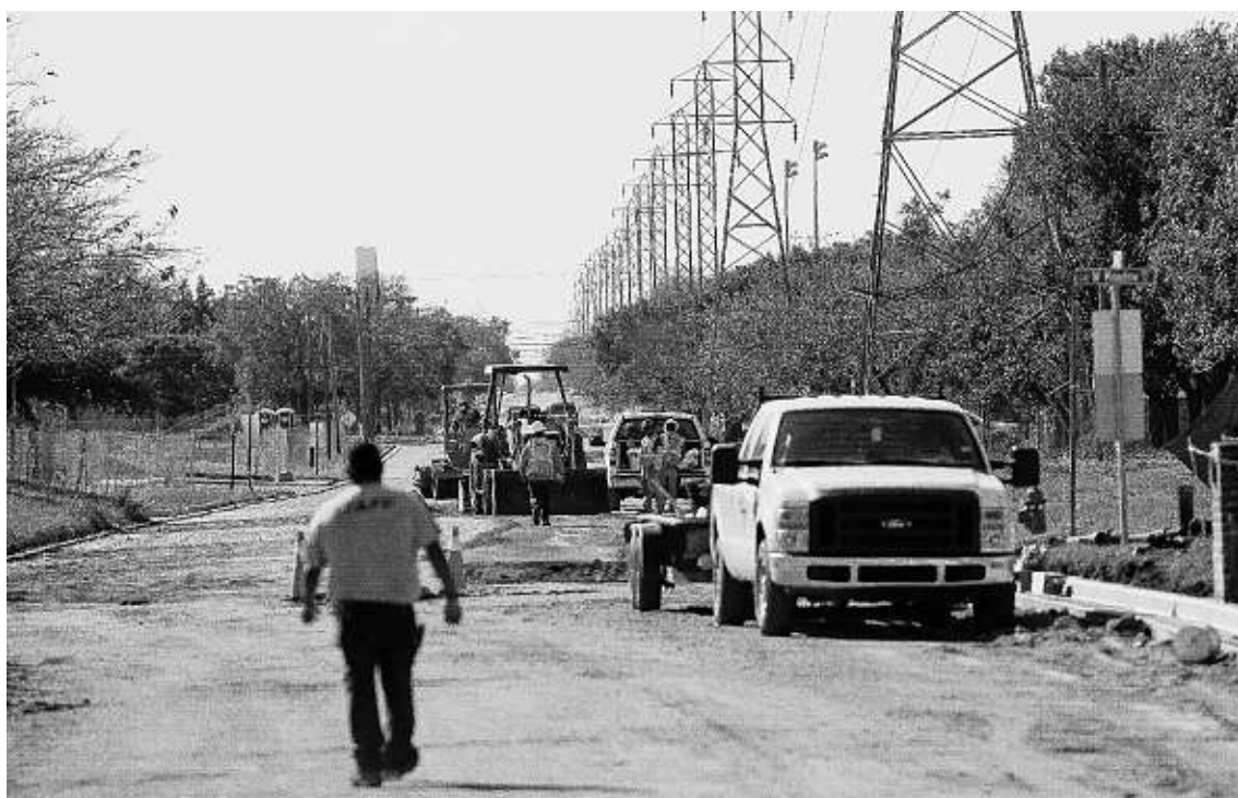
Construction workers walk down North Reagan Street in West as crews continue to repair damage to the road and pipelines.
